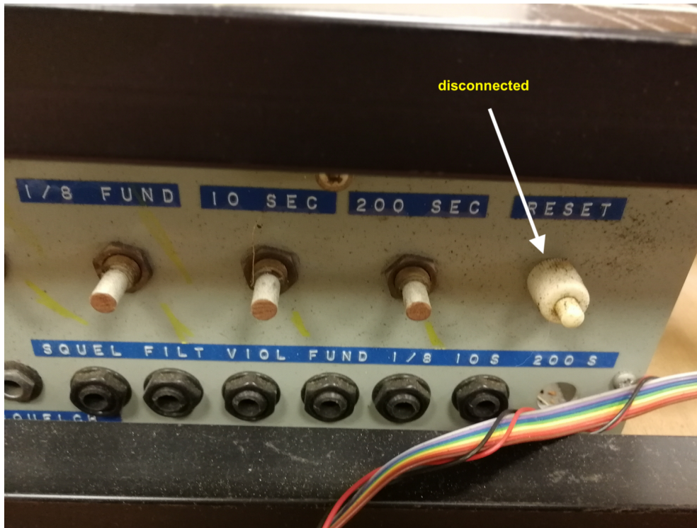
Figure 26 yet more details. The 'RESET' switch is actually disconnected. Original purpose?
